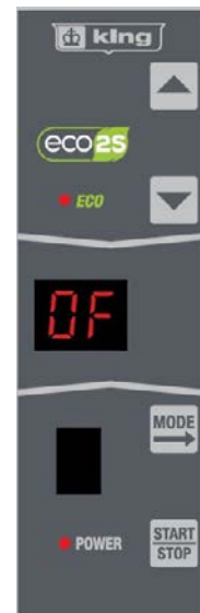
Heater Display – Heater Locked Out
