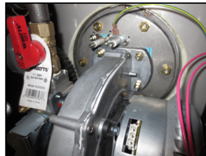
Figure 4 - Blower with Wires Removed
