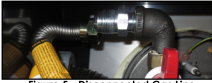
Figure 5 - Disconnected Gas Line
