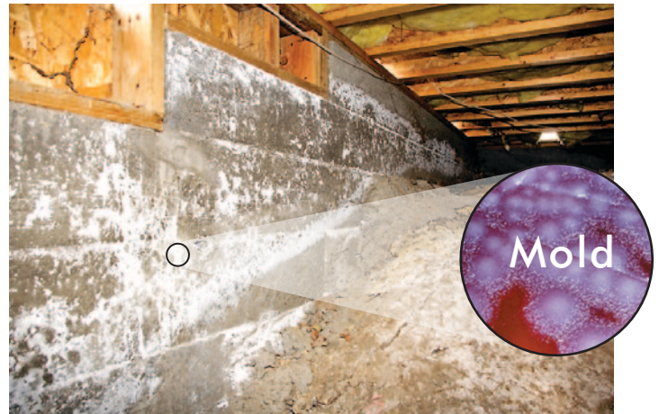
Typical crawl space under home with mold growth
