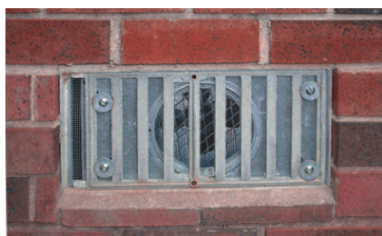
Installed behind existing vent
