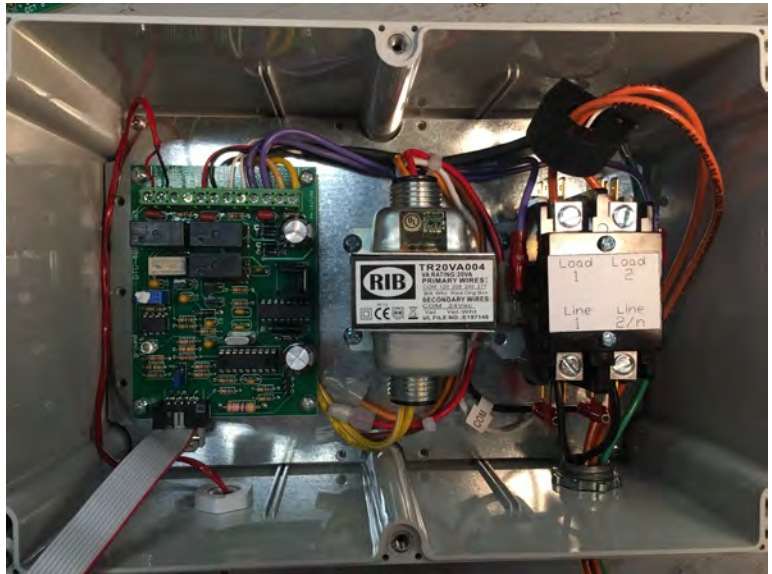
Does yours look like this? Note the load wires through the toroid coil (donut).
