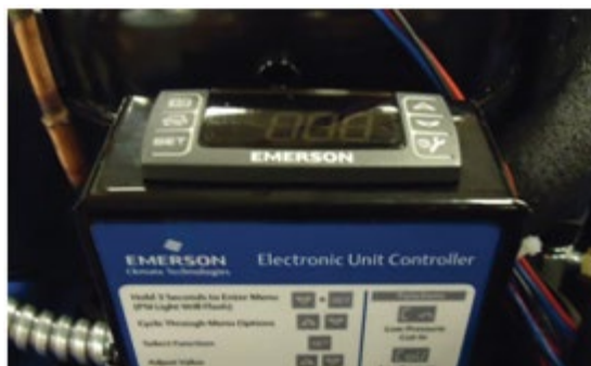
Figure 11 – Small Black Electrical Box
