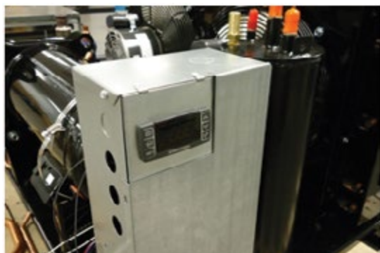
Figure 10 – Silver Electrical Box
