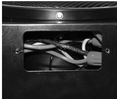
Figure 14: Wire connections carefully pushed into wiring compartment
